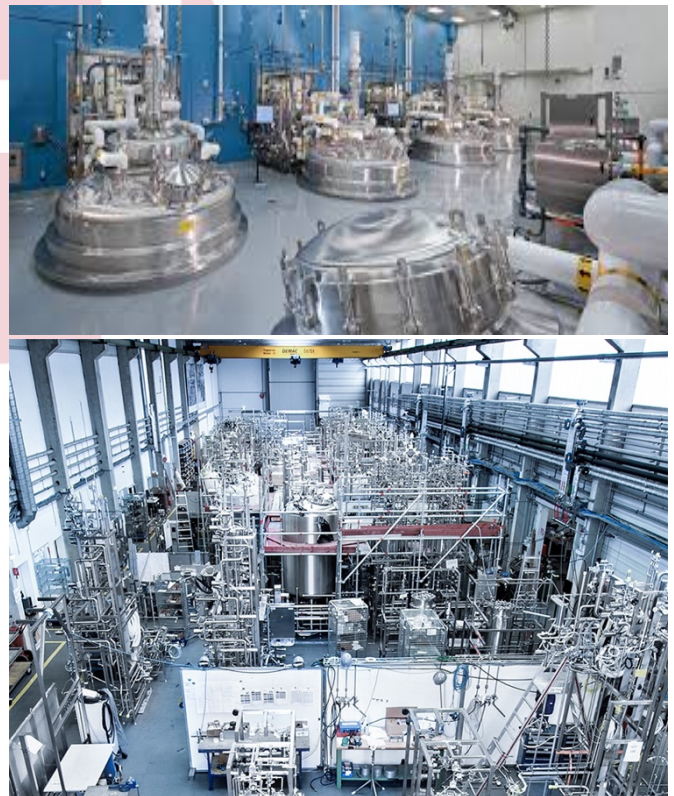
Figure 2: A large-scale biologics manufacturing suite (top), picture from DPR.com. Biologics manufacturing equipment under construction off site (bottom), picture from Zeta.com
